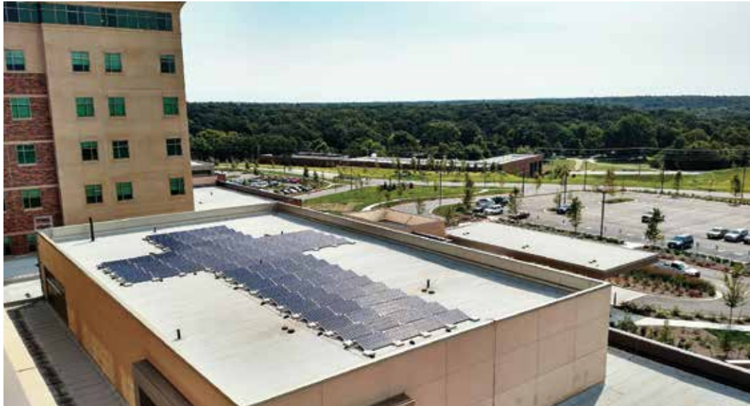
Solar panels on the roof of Mercy Hospital Joplin in Missouri.
